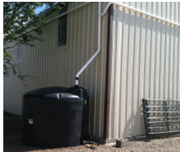
Catchment System at PGCD's Office
