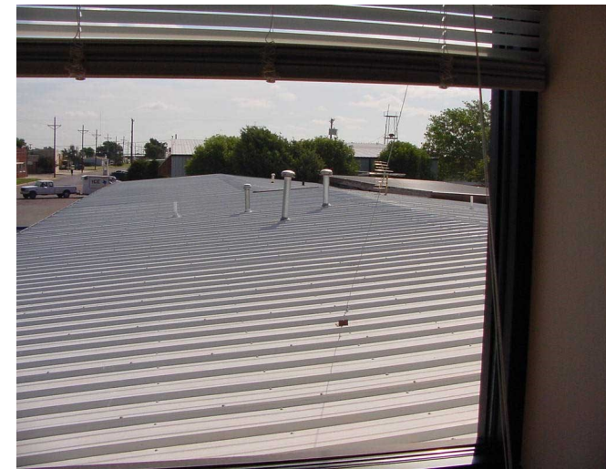
The roof of the main building at PGCD's office provides our catchment area.
